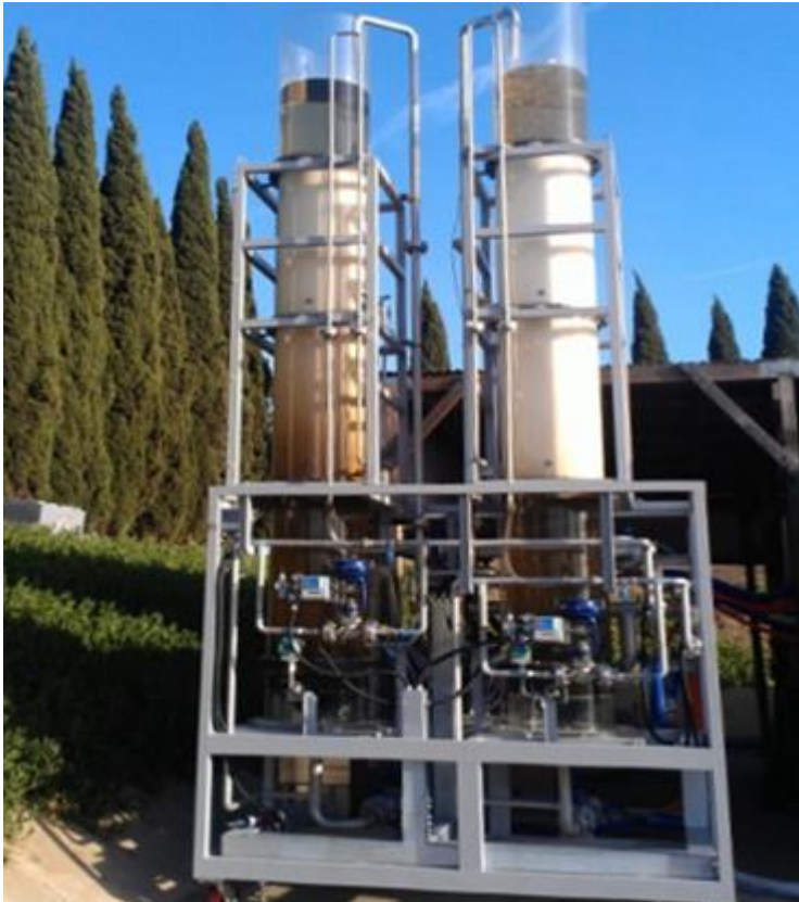
CA Title 22 Certification Testing Facility City of Carson, CA
